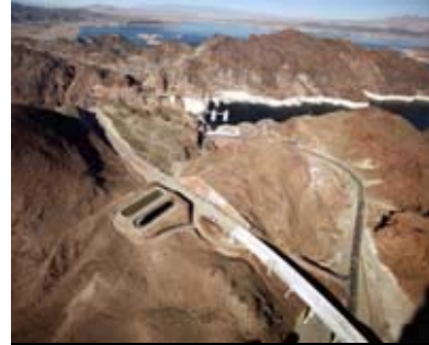
Road construction on the Hoover Dam bypass on the Arizona side on Wednesday shows the view looking north toward Las Vegas. With the Hoover Dam bypass scheduled to open in 2008, some Las Vegas developers are buying land in Arizona to build bedroom communities. The bypass should cut the commute time by about 30 minutes, real estate experts predict.
